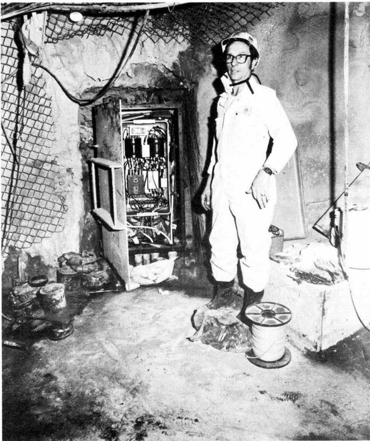
STARTLED BY THE PHOTOGRAPHER, Ray Peabody (7132) is caught in his work location, deep in a tunnel in a bypass drift next to a shot site. He's working on the arming and firing system for the MAC and GSAC gate closure systems (see Closures story). A part of Field Engineering since 1968, Ray typifies the breed: "I enjoy the work," he says. "Each shot poses different challenges, so the job never gets to be routine." Photo by Chris Salinas, REECo
